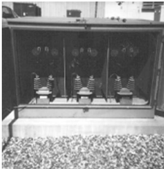
Figure 6-10. Underground primary metering. Courtesy of Alliant Energy.
