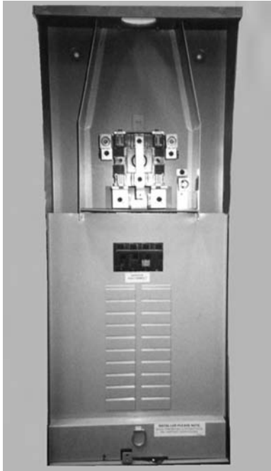
Figure 6-13. Meter cover removed.
