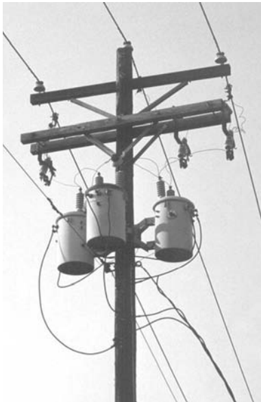
Figure 5-18. Three-phase transformer bank.
