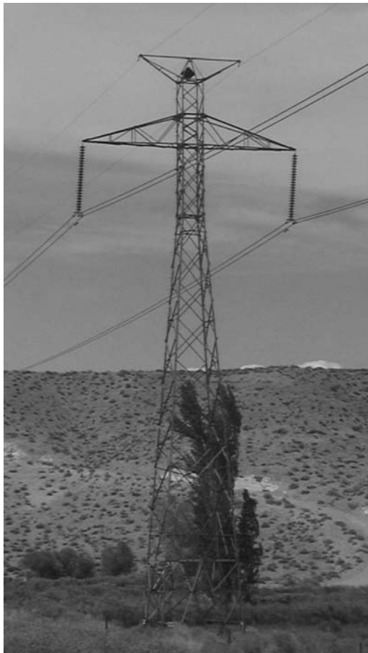
Figure 3-7. Overhead dc transmission line.
