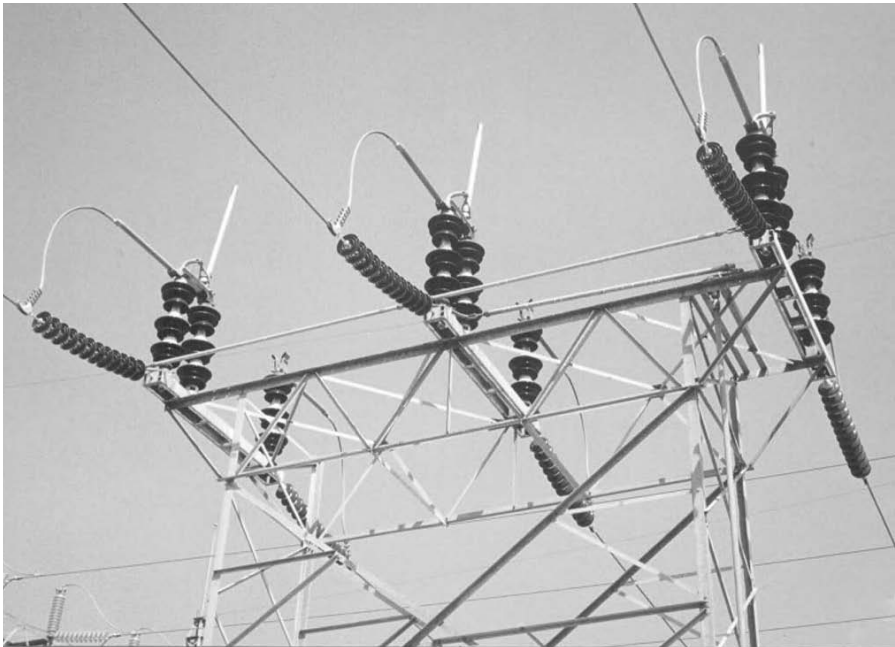
Figure 4-32. Vertical-break switch. Courtesy of Alliant Energy.
