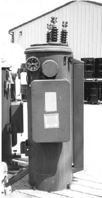
Figure 4-17. Single-phase regulator. Courtesy Alliant Energy.
