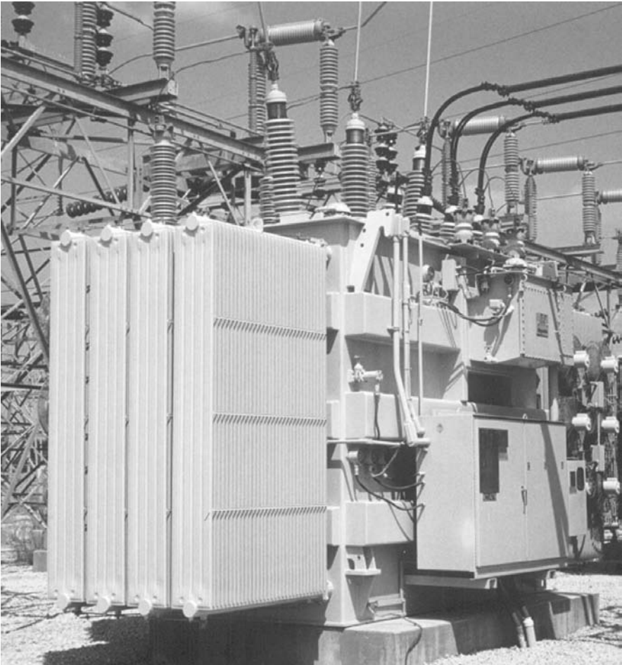
Figure 4-2. Distribution power transformer.
