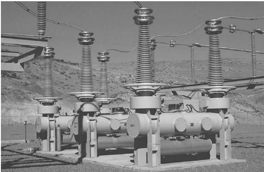
Figure 4-26. 345 kV Gas breaker.
