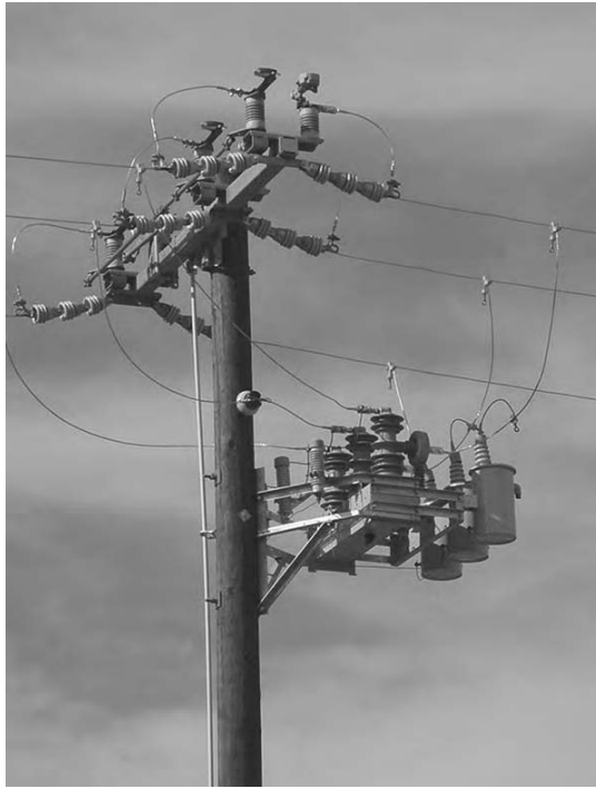
Figure 6-11. Overhead primary metering.
