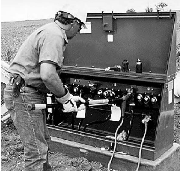
Figure 5-29. Load-break connections. Courtesy of Alliant Energy.
