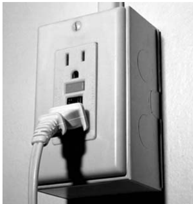
Figure 10-13. Safety hazards at home. Always be vigilant about electrical safety at home!
