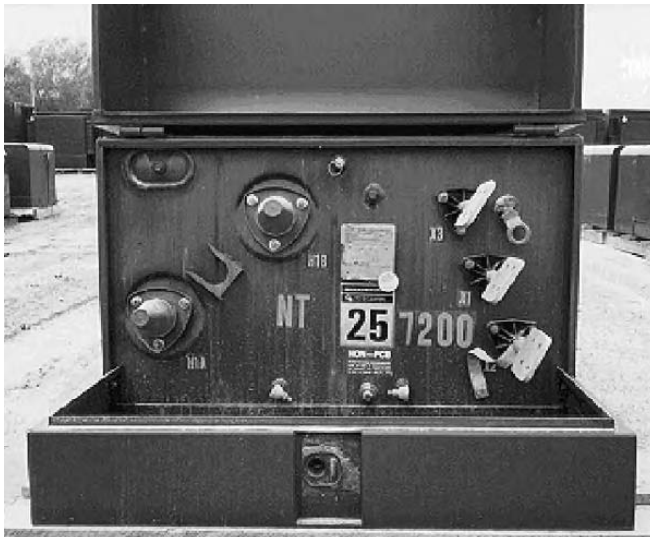
Figure 5-34. Switching transformer. Courtesy of Alliant Energy.
